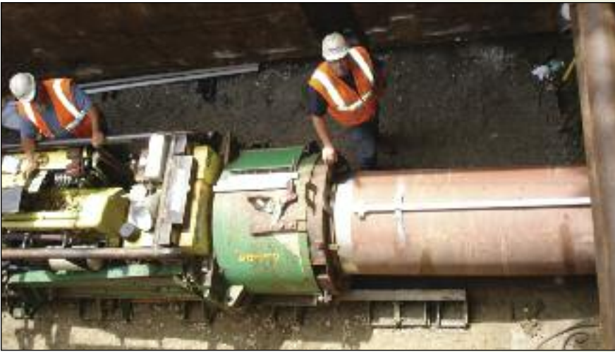
Jacking the 30-inch VCP in the final step was the smoothest part of the installation.
